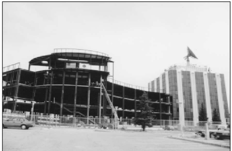
The flags of Japan and the United States mounted high on the building's structural framework signify the collaboration taking place, as construction proceeds on the new International Arctic Research Center (IARC) at the University of Alaska Fairbanks in July 1997. IARC will be physically attached to the Geophysical Institute building on the right (photo by Syun Akasofu).
