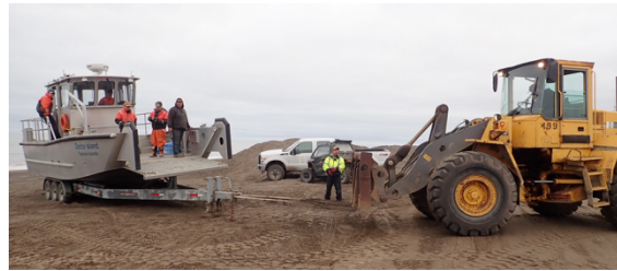
Heavy equipment being used to launch a boat big enough for large waves but too big for the boat ramp when the water is low at Utqiagvik, Alaska
